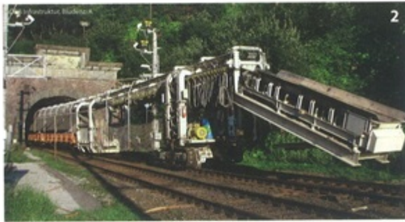
Gleiskörperabtragsvorrichtung zur Erneuerung des Arlbergtunnels Machine for removing the track superstructure during the renovation of the Arlberg Tunnel
