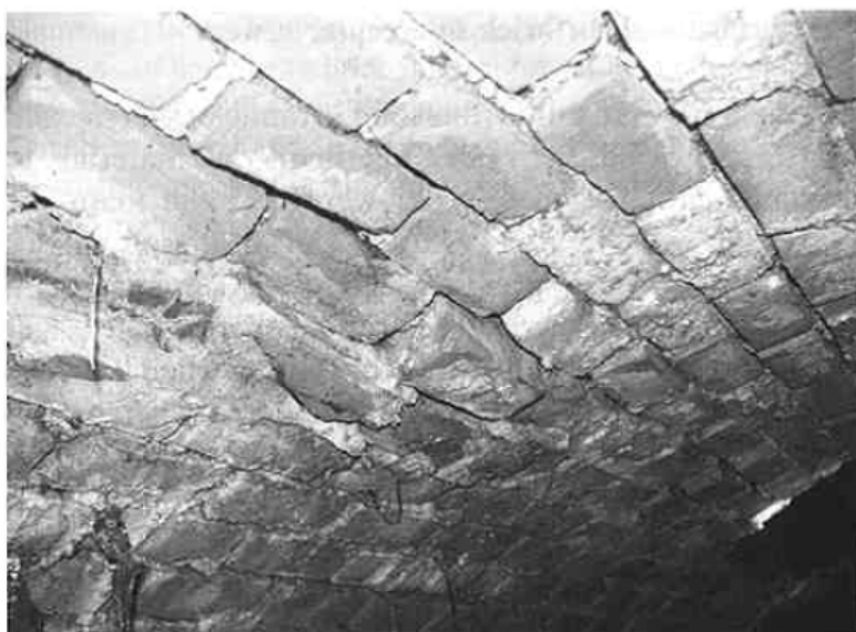
Fig. 5. Damage to interceptor sewer J – damaged mortar and dislocated bricks.
